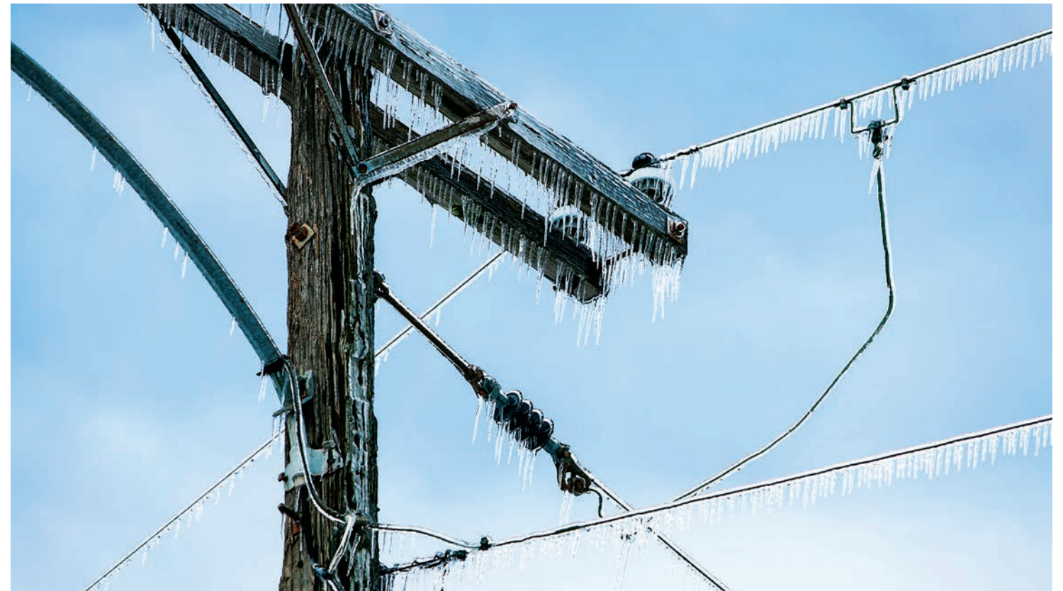
▲ Student Carlos Santana Laraquent is researching how common deicing materials can be safely applied to electrical equipment.
